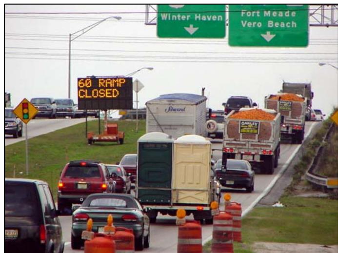
Variable message signs provide traveler information to help alleviate traffic congestion. SR 60 Bartow
